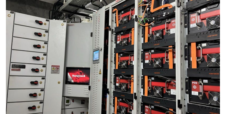
Battery Energy Storage System Project at Lakshadweep
