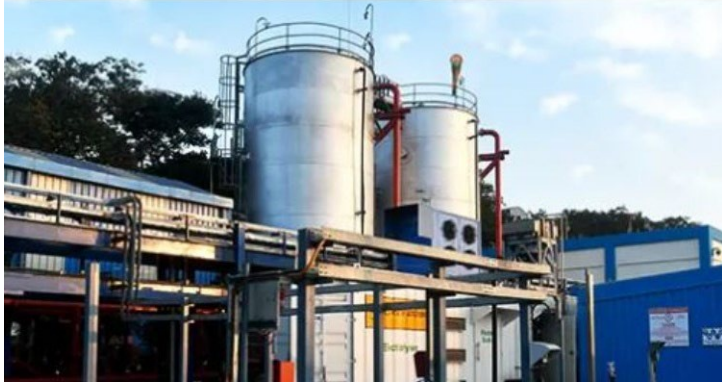
Successful implementation of automation solution for indigenously built Green Hydrogen Plant
