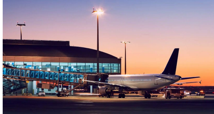
Deployment of Honeywell's advanced visual docking guidance system (AVGDS) at an airport in India
