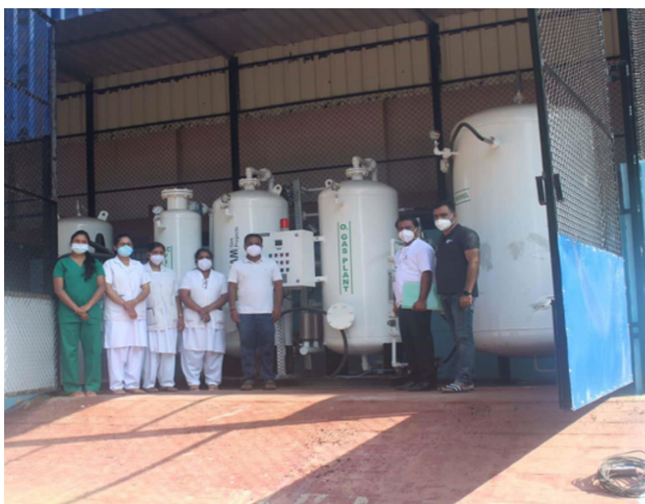
Oxygen Generation Plant at Karnal, Haryana
